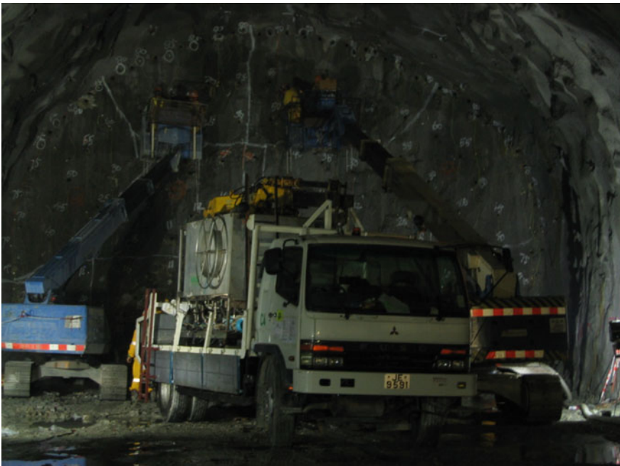
Fig. 16.20 AMSHK's emulsion pump truck is charging in tunnel face (courtesy of AMSHK)
