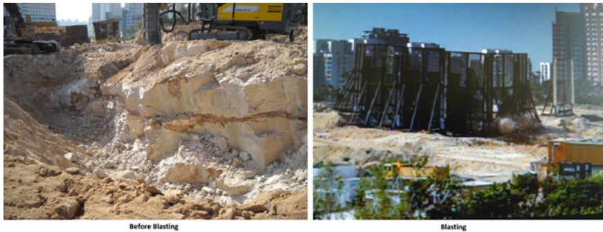
Fig. 1.37 An open joint in rock mass caused high airblast in project DAR, HK, 2009
