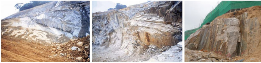
Fig. 1.41 Slope failure by discontinuities
