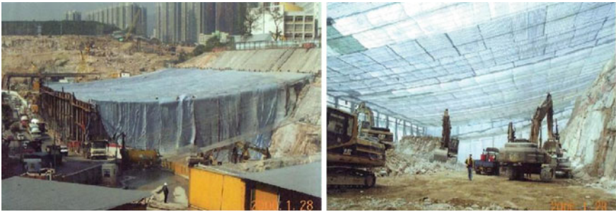
Fig. 11.13 Roofover protective structure for MTRC Yau Tong Station of Hong Kong. Left external view; Right inner view
