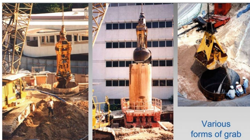
Fig. 14.36 Borehole formed by chisel and grab and support with casing. (Reproduced from Ref. [16] by permission of City University of Hong Kong)
