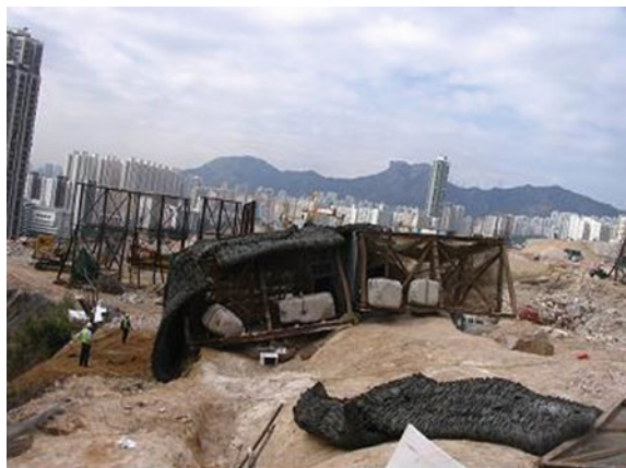
Fig. 11.33 Thick rubber tire mats covering on the top and side of the cages which is facing to the residential buildings
