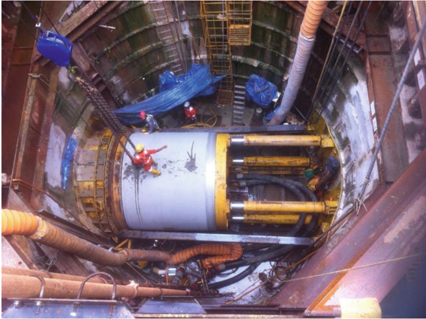
Fig. 15.10. Pipe jacking operation in the driving shaft (reproduced with the permission from Ed. Züblin AG—Singapore Branch)
