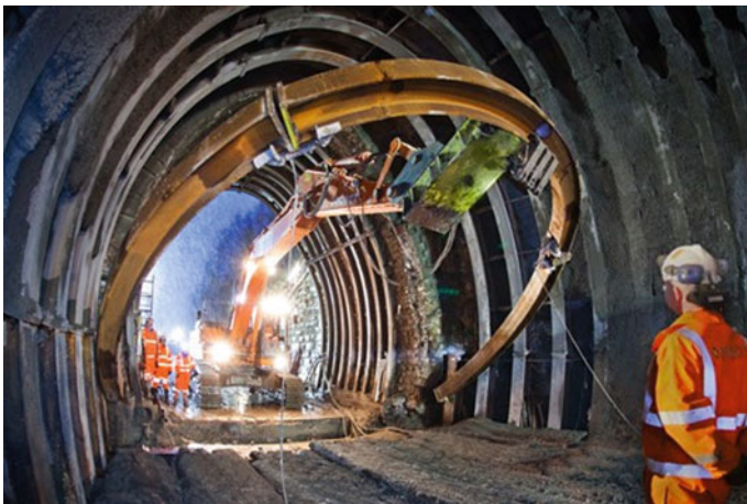
Fig. 21.43 The old steel arches of Holme Tunnel were replaced with new arches Source www.railmagazine.com
