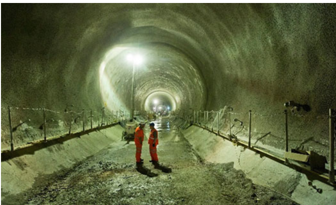
Fig. 21.41 A second mass-pass-transit cross-rail line in London lined with shotcrete Source www.theguardian.com/uk/crossrail
