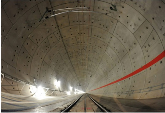
Fig. 21.44 Segment lining system support the ground with a structure made up of a number of preformed interlocking elements
