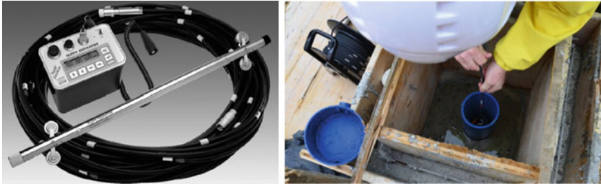
Fig. 22.11 Vertical inclinometer and inclinometer measurement
