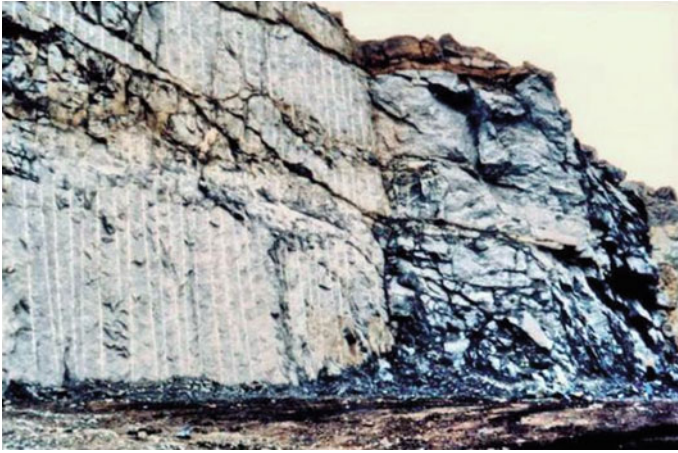
Fig. 10.1 Comparison between the results achieved using control blasting ( on the left ) and normal bulk blasting for a surface excavation in gneiss
