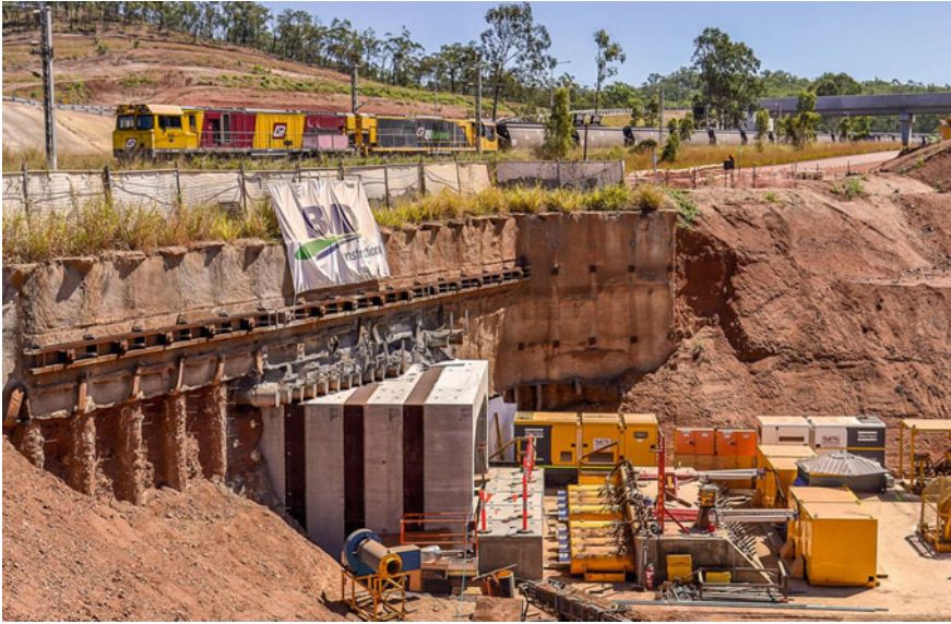
Fig. 15.7. Box culvert during Jacking operation under rail line at Wiggins Island Coal Export Terminal Gladstone, Qld Australia (Reproduced with the permission from Tunnelcorp Pty Ltd.)
